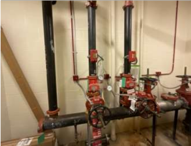
19 - FIRE SUPPRESSION SYSTEM
