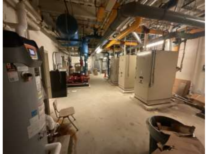
8 - MAIN MECHANICAL ROOM
