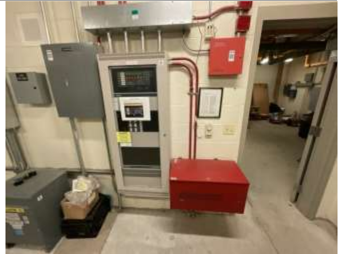
20 - FIRE ALARM SYSTEM
